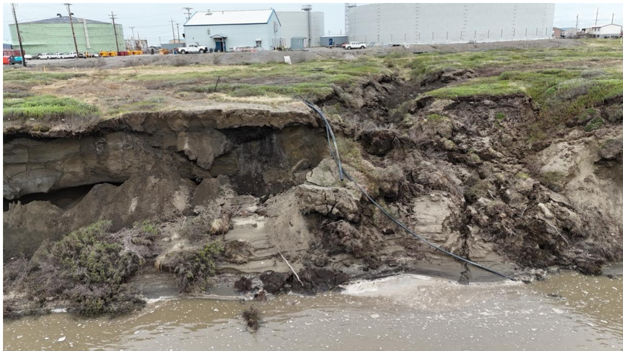
Figure C.3. Drone imagery of the original site area following spring breakup, showing active bank collapse and exposed infrastructure. Significant thaw-related slumping occurred along the channel edge. (NVN DNR, 2025)
