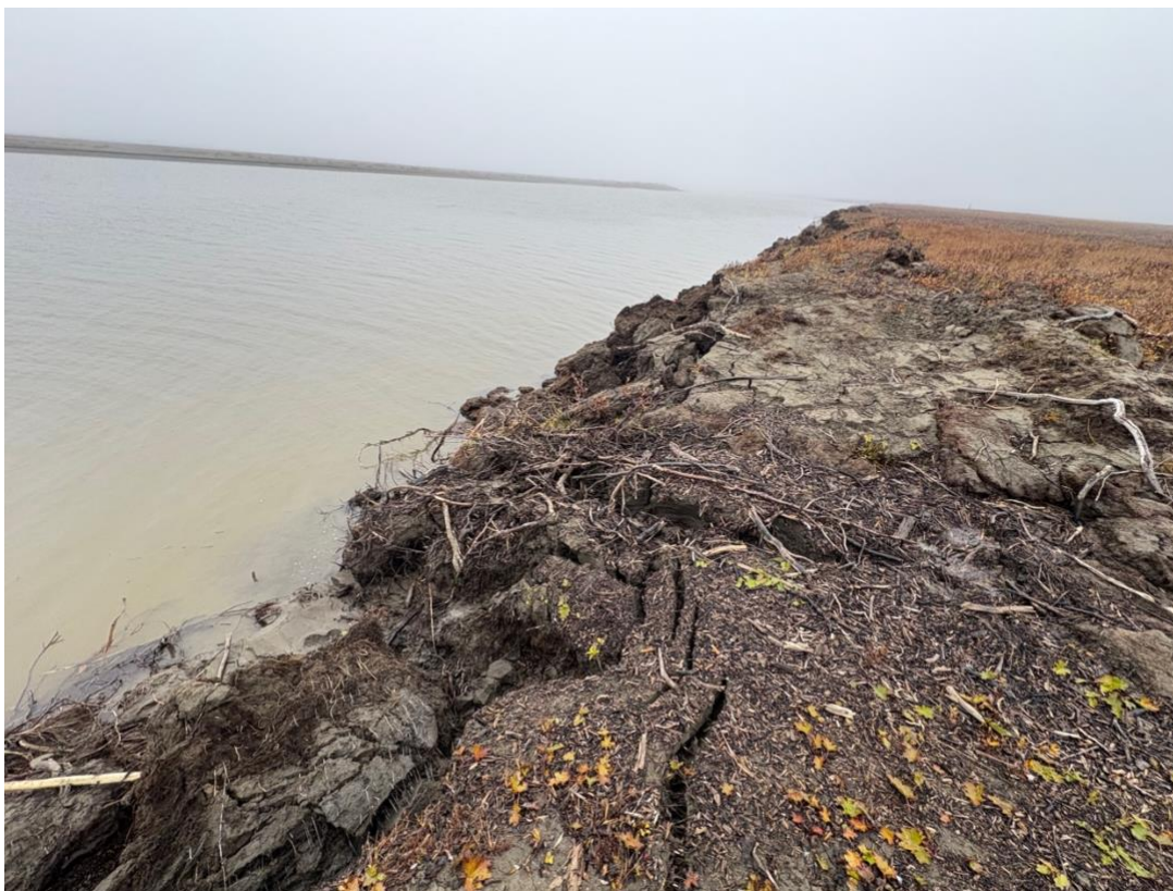
Figure C.20. Riverbank erosion and cracking above the monitoring site after floodwaters receded. (NVN DNR, 2025)
