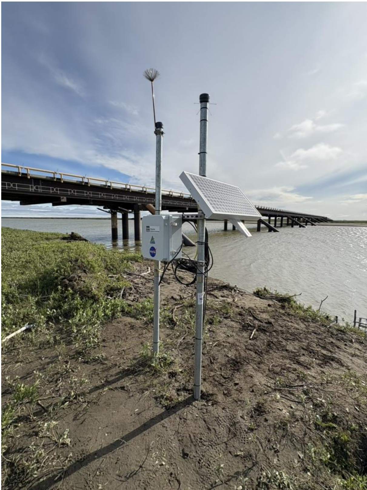
Figure C.16. Final installed monitoring station showing solar array, antenna, and telemetry housing in operational configuration. (NVN DNR, 2025)
