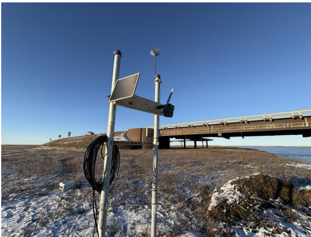
Figure C.29. Site overview showing the decommissioned telemetry station and newly installed monitoring camera with solar array on the upper bank, which will be used to remotely monitor the site over the winter season. (NVN DNR, 2025)
