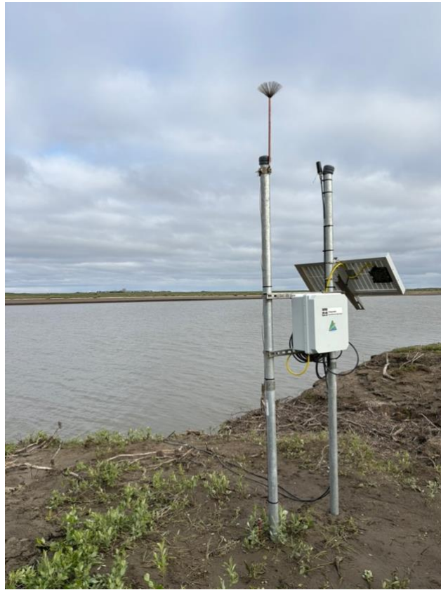
Figure C.12. Solar-powered telemetry and logging system following completion of installation, facing east across the Niquiq Channel. (NVN DNR, 2025)
