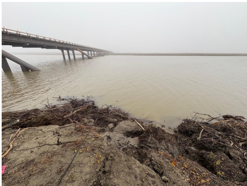
Figure C.23. Overview of the Niquiq Bridge and adjacent bank slumping, along with almost completely submerged sensor ladder, after the August 2025 high-water event. (NVN DNR, 2025)
