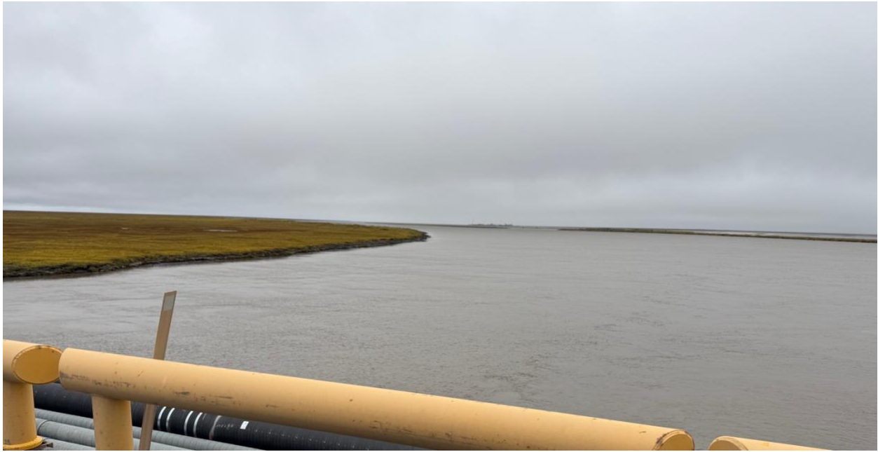
Figure C.18. View from the Nigliq Bridge showing elevated channel levels during late-season flooding. (NVN DNR, 2025)
