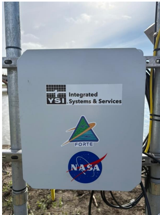
Figure C.11. Close-up of the system enclosure showing NASA FORTE and YSI Integrated Systems & Services identification labels. (NVN DNR, 2025)
